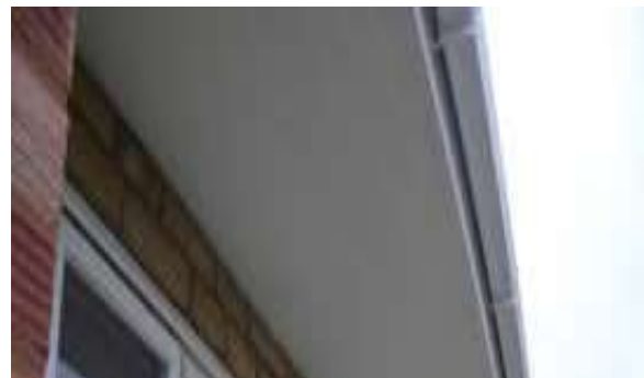
Pieces of Asbestos Insulating Board (AIB)
