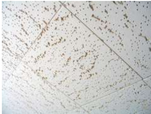
Asbestos containing ceiling tiles
