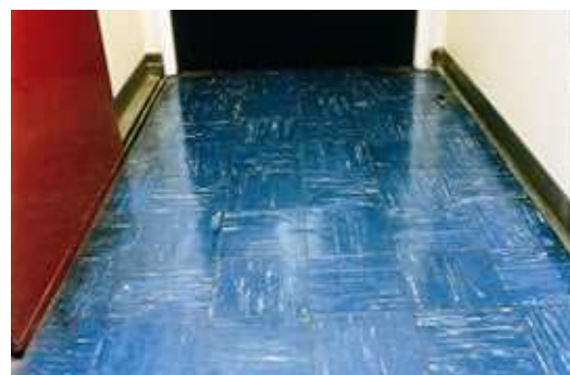
Asbestos containing floor tiles in a corridor
