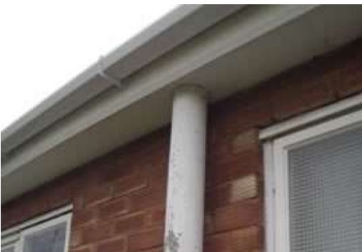
Asbestos cement drainage pipe (downpipe)
