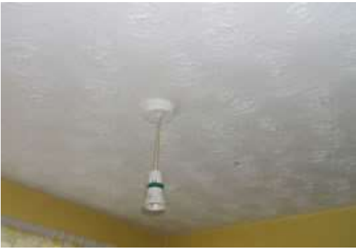
Asbestos textured coating
