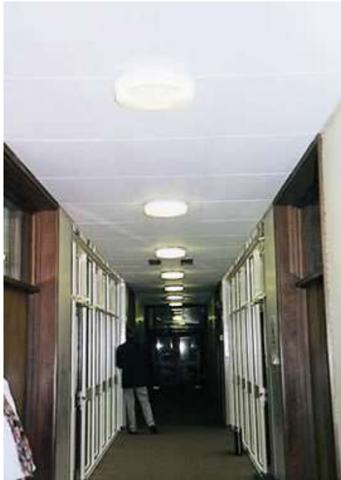
Suspended Asbestos Insulating Board tiles in a corridor
